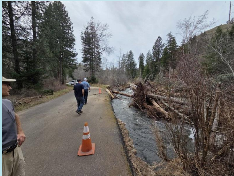
Road Damage between Camp Wooten and USFS Tucannon Campground
