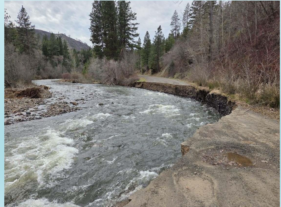
Road wash-out in March 2026 flood near Camp Wooten
